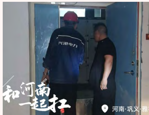
▲ 4:00 am The employees of CIFI Ever Sunshine were checking power distribution equipment all night in the community
