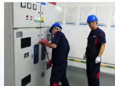
▲ Project power supply and distribution inspection
