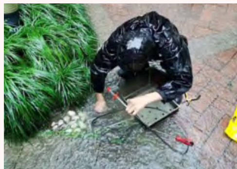
▲ Inspection and unblocking of the facilities and drainage network in the community, building flood control walls at garages and low-lying entrances and stock emergency materials
